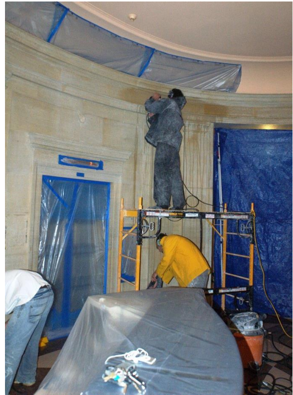
(Image Above) Extensive protection of adjacent wall surfaces was required to minimize any impact from overspray. (Below) Worker honing the wall surface with a hand-held polisher.
